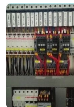
MCC & motor control
