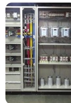
PFC / capacitor banks
